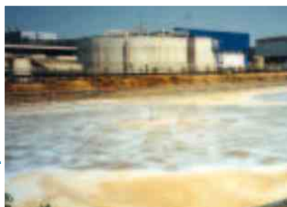
Submersible aerators type SCL installed in a wastewater treatment plant
